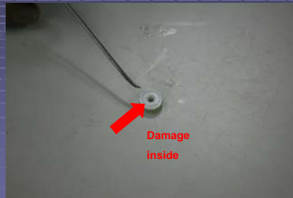
Check any damages of Valve and O-ring
